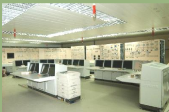
Main Control Room KKNPP-1
