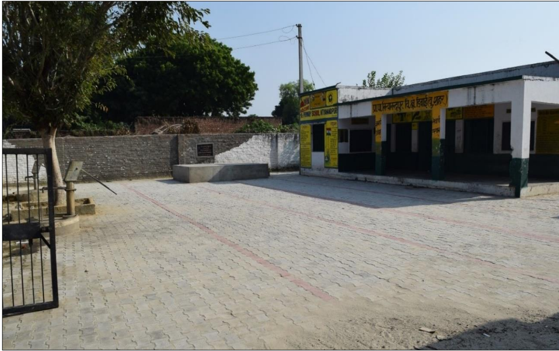
Construction of flooring in open area and platform at Primary School, Nandpur, Uttar Pradesh
