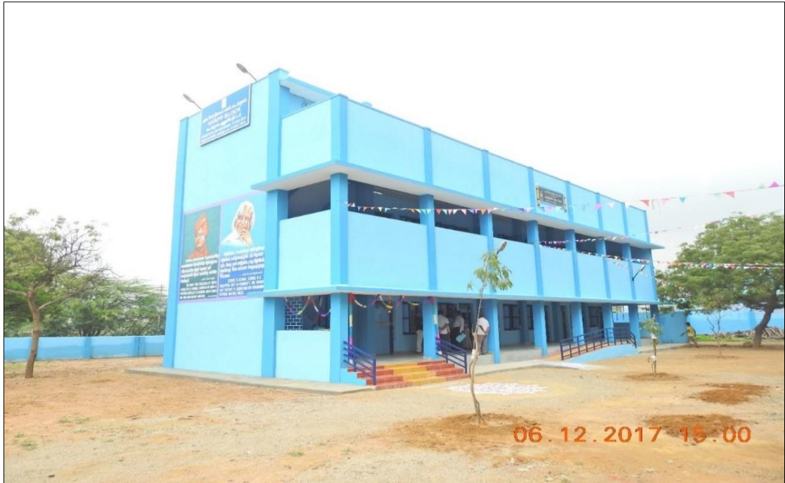
Construction of additional class room building and science lab. at Kudankulam, Tamil Nadu
