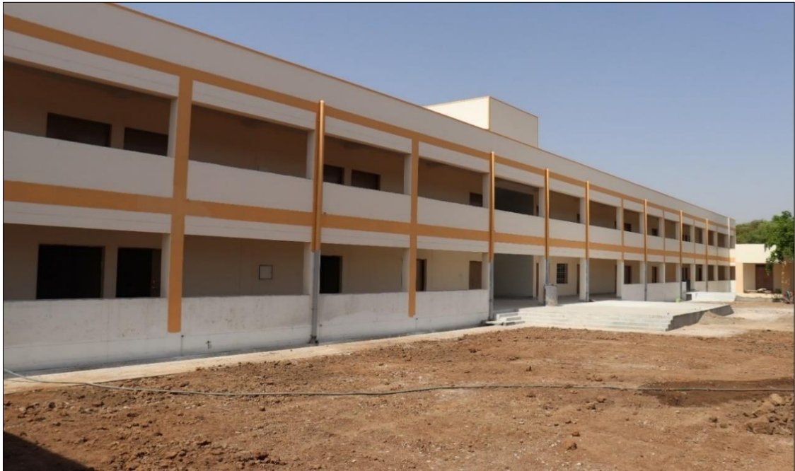
Construction of new school building at Government Senior Secondary School Eklingpura, Rajasthan
