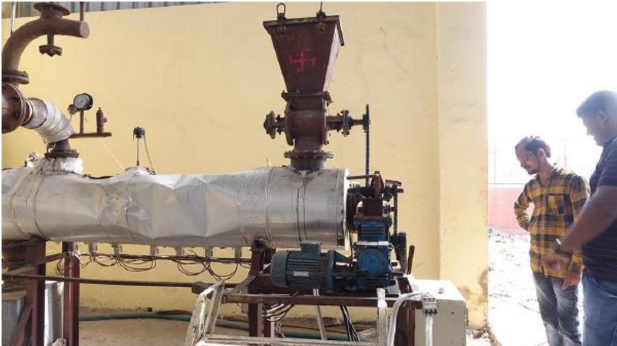
Resource recovery station cum solid waste management plant at Vyara, Gujarat
